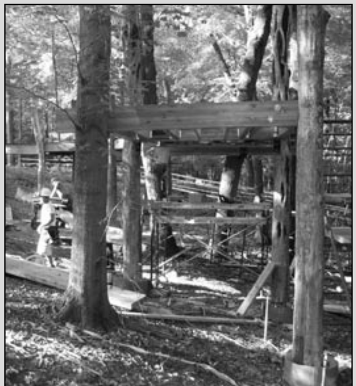
The structure is supported by white oak, red oak, sugar maple, and black walnut trees and black locust support posts. The brackets that attach the treehouse to the living trees are specially designed to allow movement and growth of the trees. The bolt that is drilled into the tree is made of titanium.
